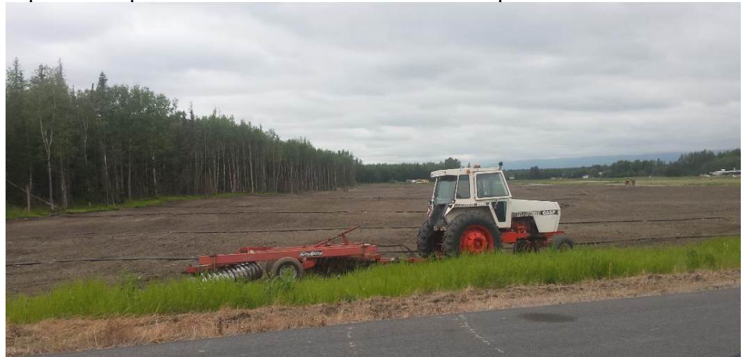
(Photo: Cleared transitional surface off RW 10/28 ready for brome hay seeding looking west)
