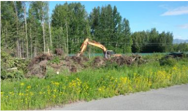
(Photo: Tree Clearing and Excavation on the Lazy Mountain Hangar Project Begin in Late June)
