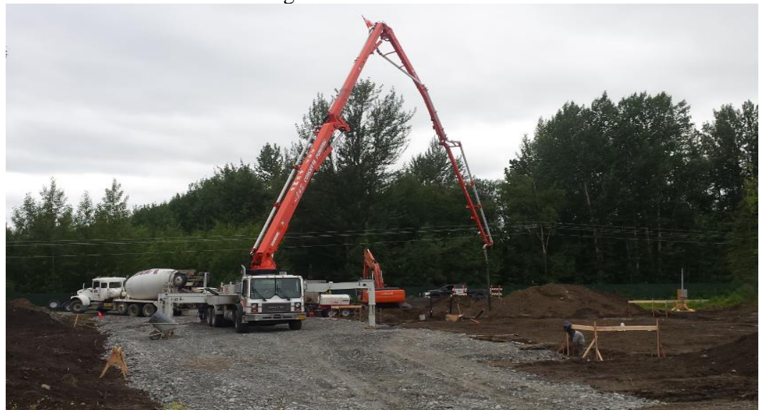
(Photo: An S & S Concrete Pump Truck Places Concrete inside of Footings July 9 th , 2020)
