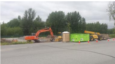
(Photo: Equipment is Staged for the Next Days Activities of Footing Excavation)
