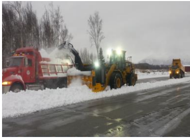
(Photo: Cleaning up the windrowed snow berms on the back side of Apron A)
