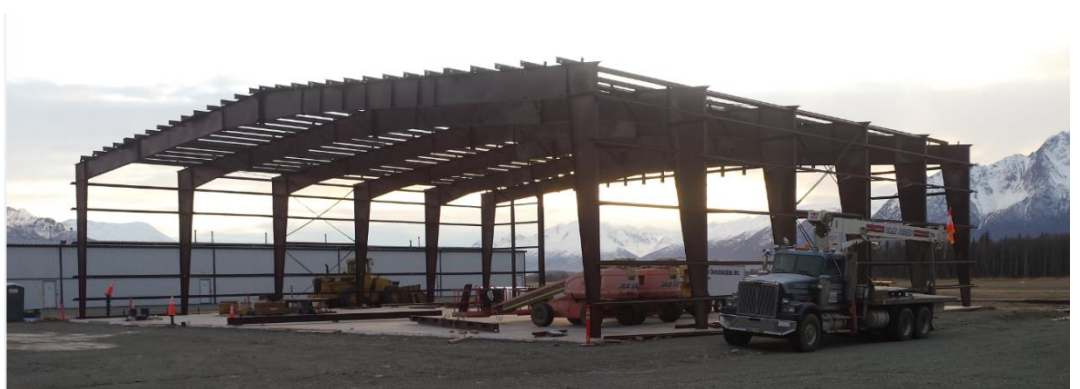
(Photo: The building is almost ready for its outside wall skin and roof panels)
