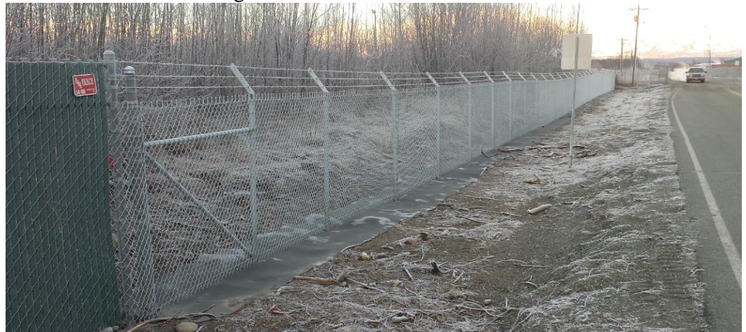
(Photo: Completion of new fencing installed along S. Airport Rd in route to the Flight Service Center building)
