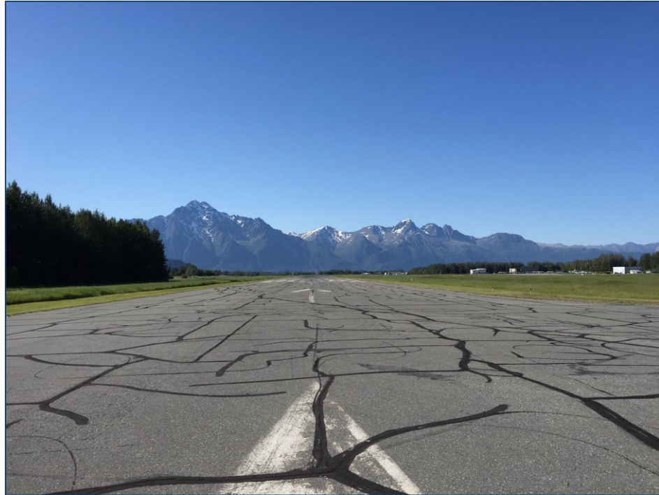
Photo: Many sealed cracks in Runway 16/34.
