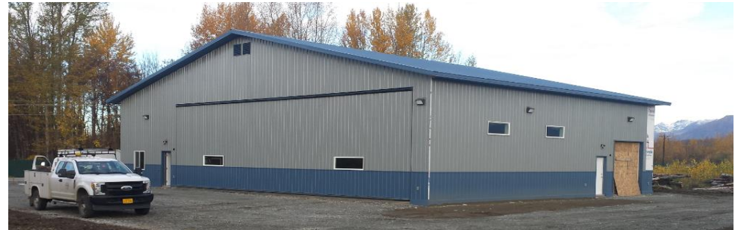
(Photo: Finishing details: The siding on this 60' X 80' hangar is almost completed, October 5, 2020)
