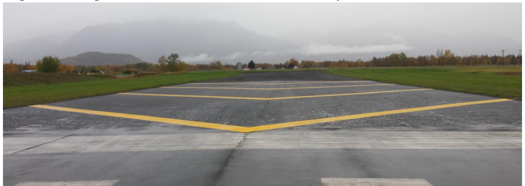
(Photo: The completed blast pad paving looking south departure path off RW 16)
