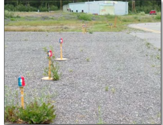
Figure 2-17. Threshold Lights (Runway 9 end)
