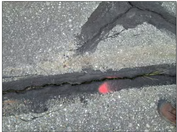
Figure 2-15. Pavement Cracks (Severity)
