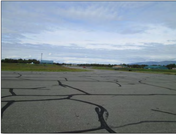
Figure 2-14. Pavement Cracks (Magnitude)
