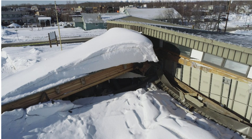
Photo 3: Roof Snow Drift
