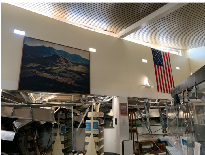
Photo 7: Collapsed Framing and Remaining Soffit
