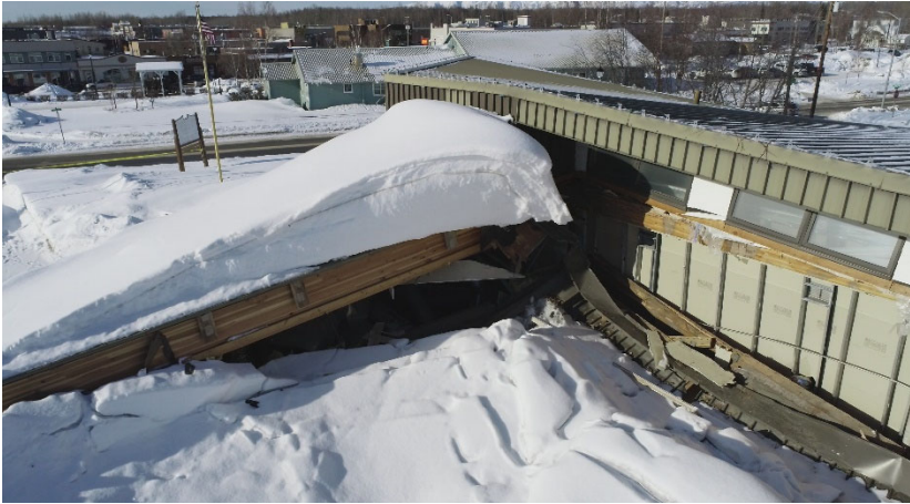
Photo 3: Roof Snow Drift
