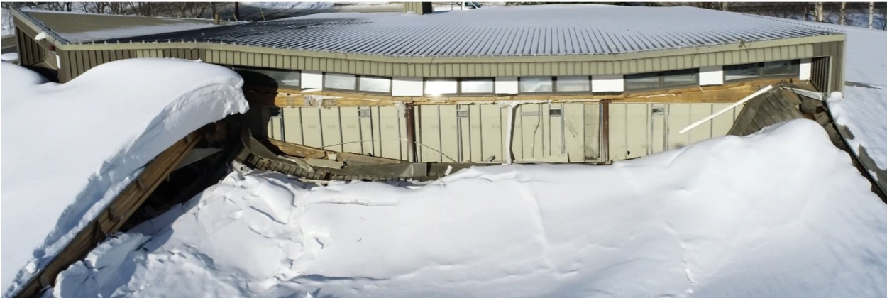
Photo 1: Elevation of Roof Collapse
