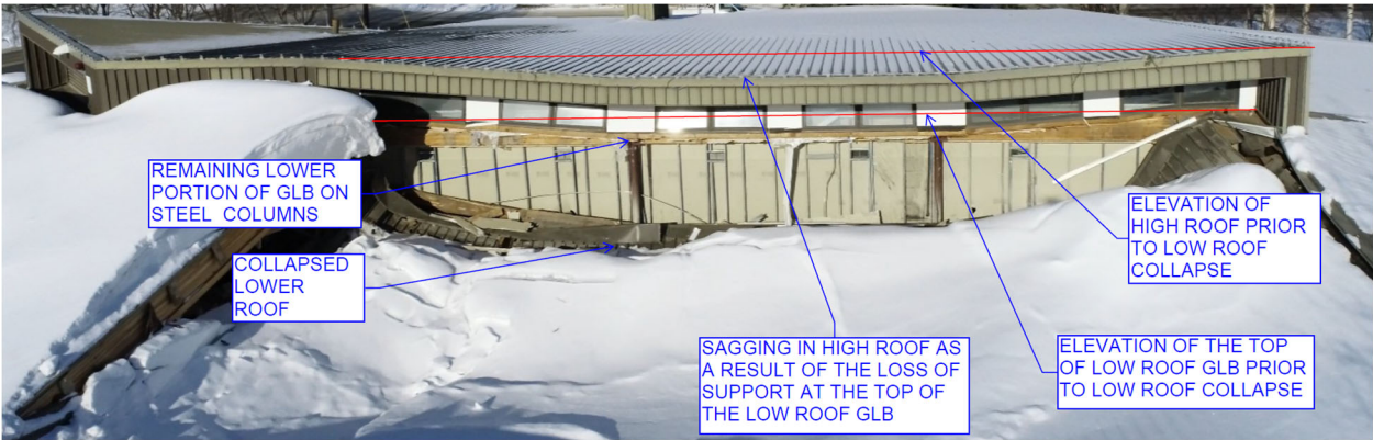
Photo 2: Annotated Elevation of Roof Collapse
