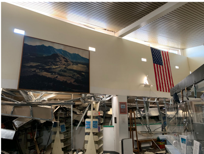
Photo 7: Collapsed Framing and Remaining Soffit
