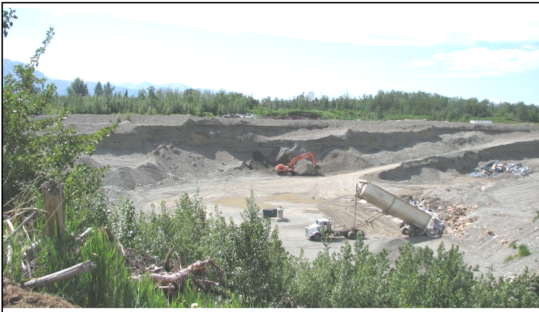
Looking southwest at Reclamation Pit fill operations from near the east side of the property.
