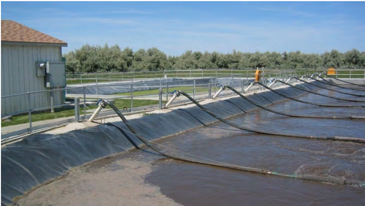
Figure 14 Aeration Strips and Blower Building at a Biolac® System
