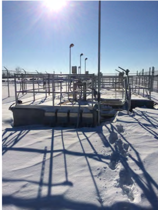
Figure 32: Cold Weather (-21F) MBBR Installation in Wisconsin
