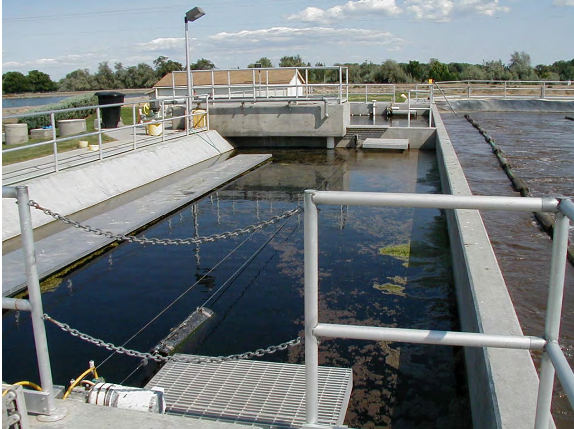
Figure 15 Secondary Clarifier with Adjacent Biolac® Lagoon.
