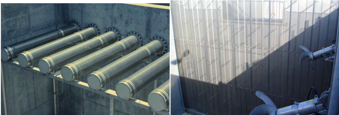
Figure 22: MBBR Media Retention Screens
