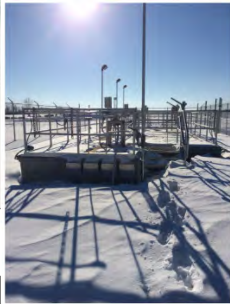
Cold Weather (-21°F) MBBR installation in Wisconsin
