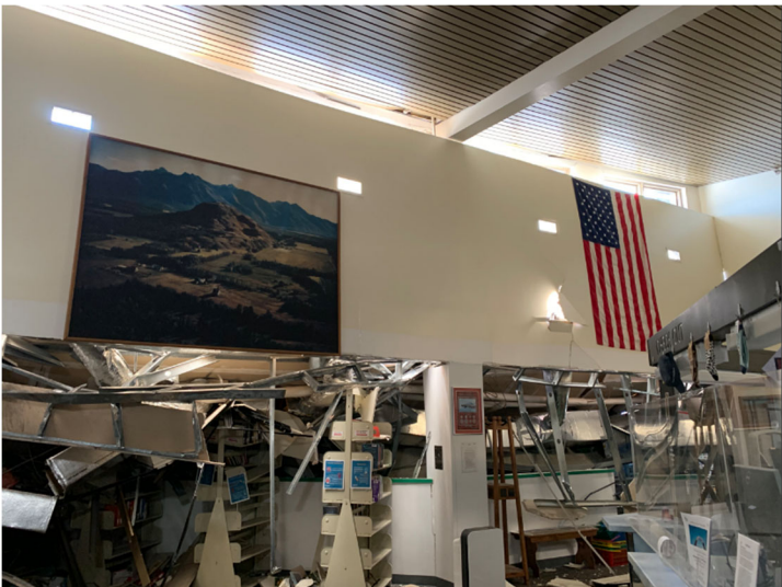
Photo 7: Collapsed Framing and Remaining Soffit
