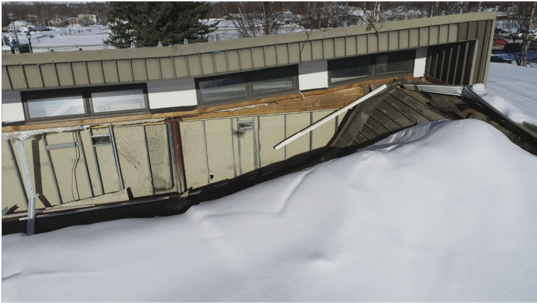
Photo 9: Damaged Steel Column
