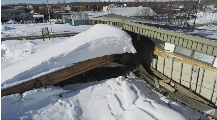
Photo 3: Roof Snow Drift
