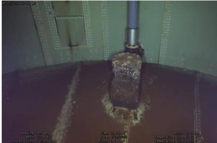
Figure 11: Inlet/outlet piping and check valve
