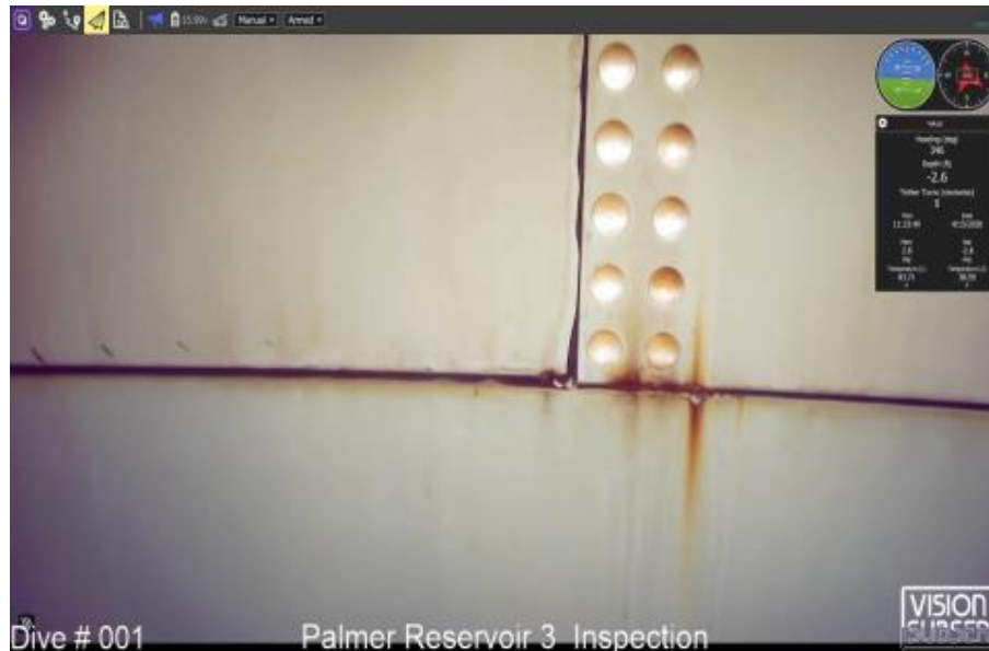
Figure 14: Typical seam corrosion
