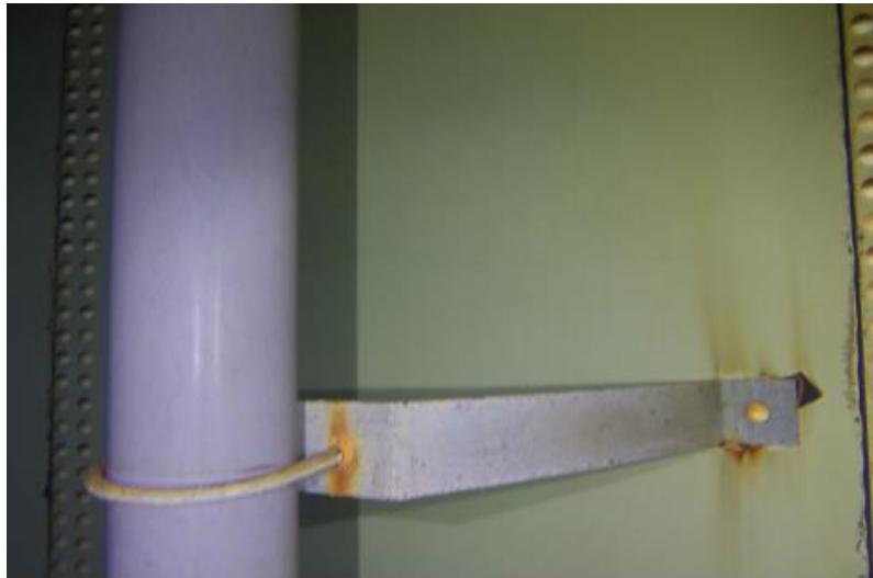
Figure 13: Inlet pipe support
