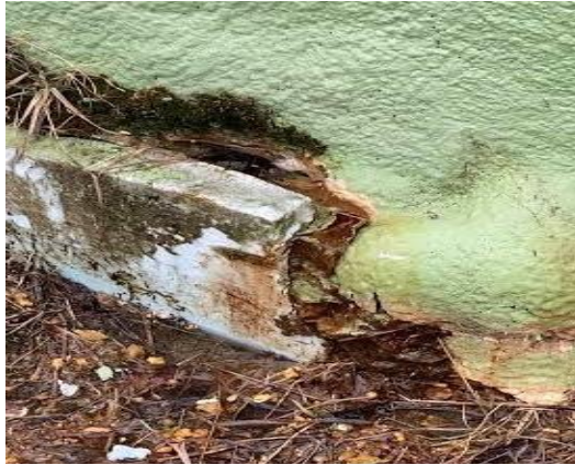
Figure 3: Reservoir leakage at tank exterior
