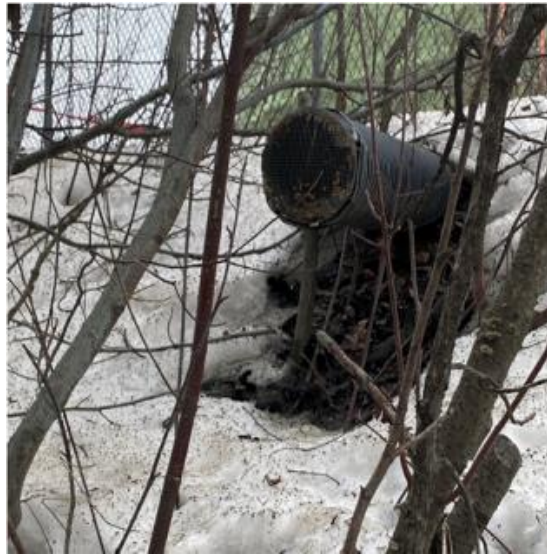
Figure 5: Overflow pipe discharge
