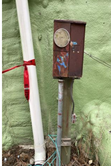
Figure 10: Electrical service meter
