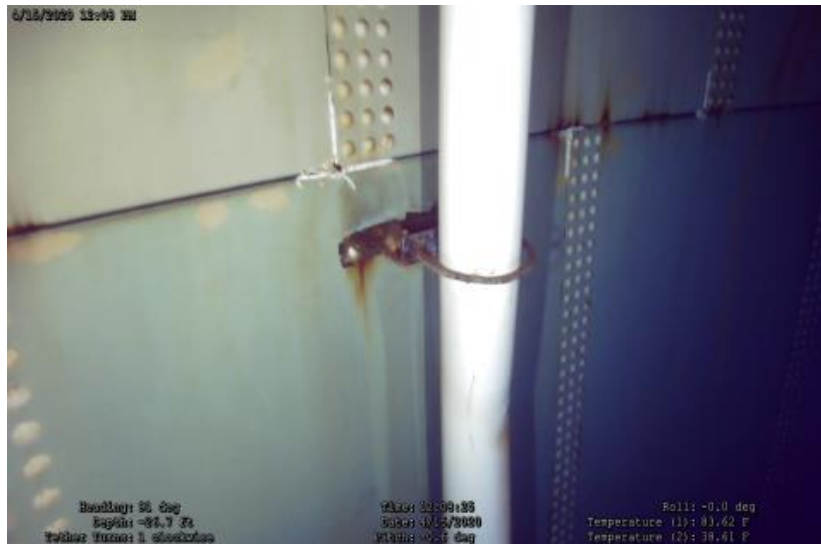
Figure 22: Decommissioned overflow to tank connection
