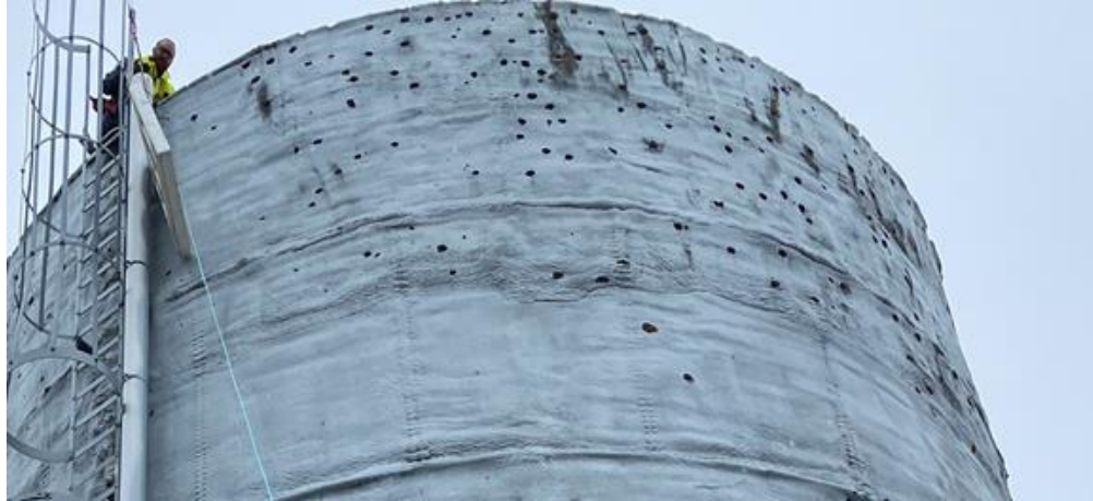
Figure 1: Insulation damage from birds
