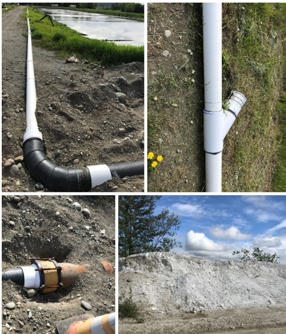
Figure 3 (Clockwise from top left): 6" PVC Dredged Solids Line along the bank of Lagoon 2; Wye connection detail (typical); Lime deposit adjacent to sludge drying area; and connection from 6" PVC Dredged Solids Line to 8" DI Dredged Solids Line (buried).
