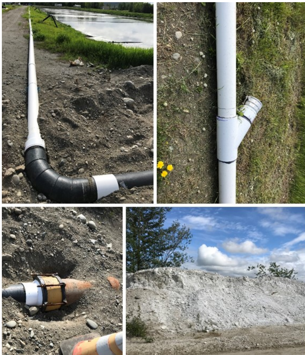
Figure 3 (Clockwise from top left): 6" PVC Dredged Solids Line along the bank of Lagoon 2; Wye connection detail (typical); Lime deposit adjacent to sludge drying area; and connection from 6" PVC Dredged Solids Line to 8" DI Dredged Solids Line (buried).
