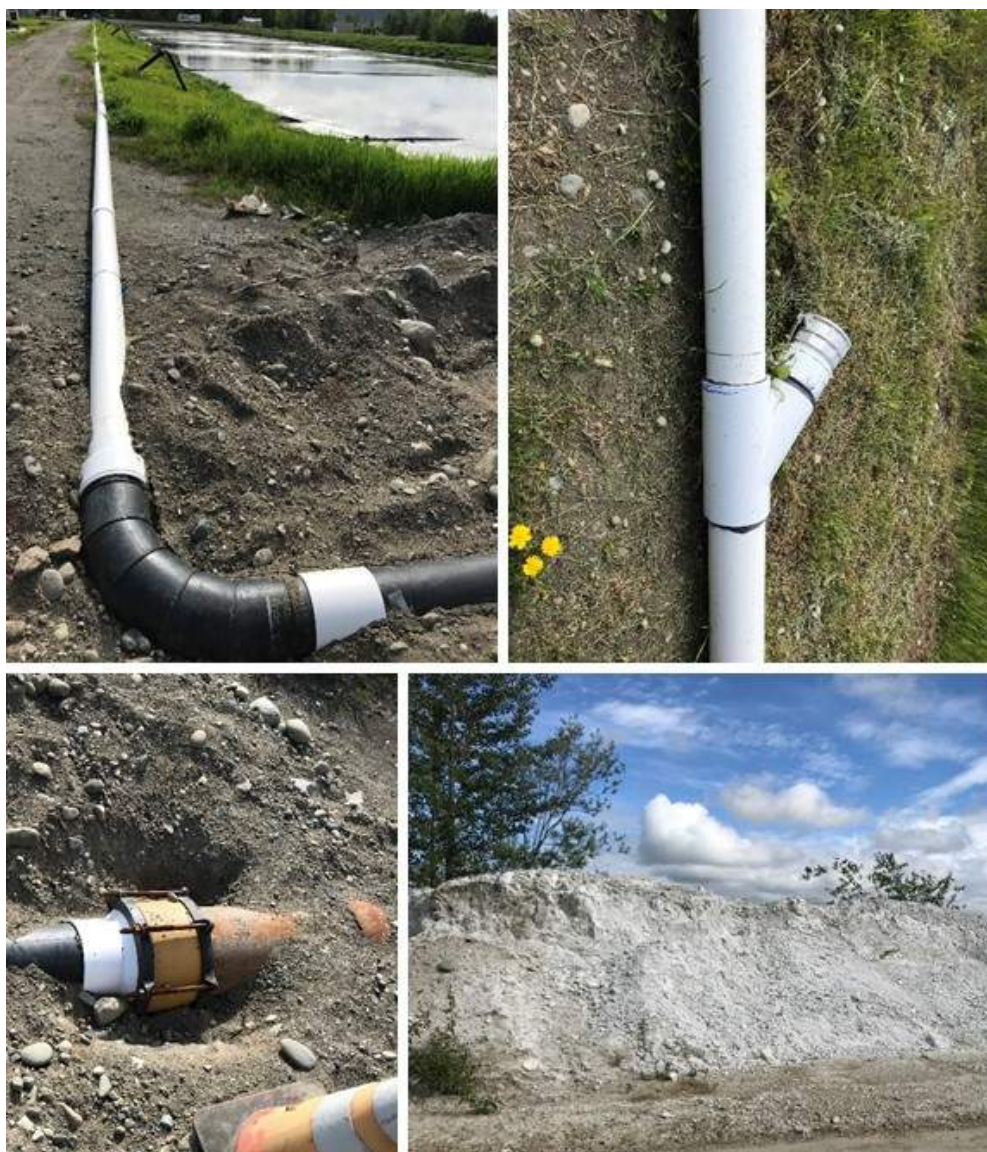
Figure 3 (Clockwise from top left): 6" PVC Dredged Solids Line along the bank of Lagoon 2; Wye connection detail (typical); Lime deposit adjacent to sludge drying area; and connection from 6" PVC Dredged Solids Line to 8" DI Dredged Solids Line (buried).
