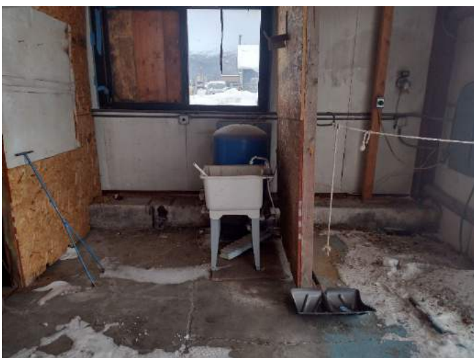
Photo 5. Boiler and Sink
