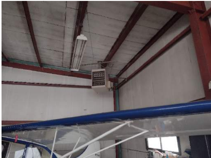
Photo 3. Overhead Natural Gas Heater in Warehouse
