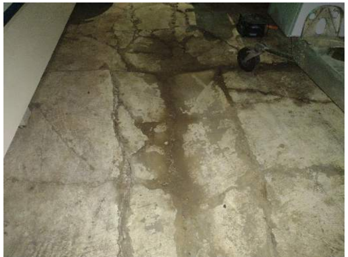
Photo 8. Staining and Cracking on Concrete Floor
