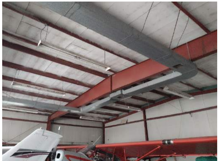
Photo 4. Venting for Former Heating System
